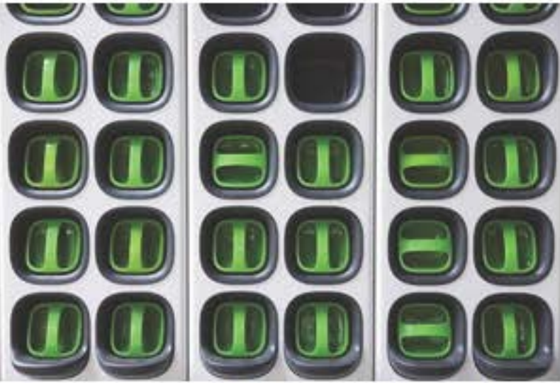
Batteries are seen at a battery-swapping station by Taiwanese electric scooter maker Gogoro Inc in Taipei, Taiwan April 19, 2022.
