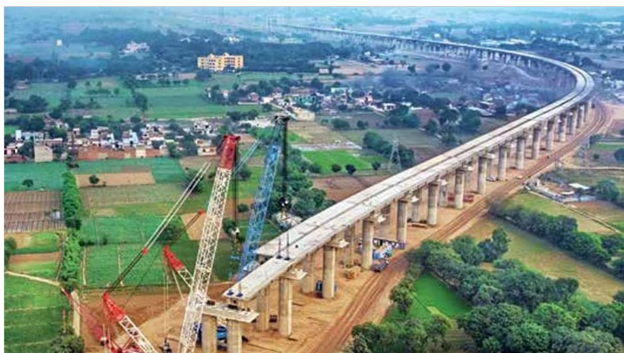
The infra thrust through dedicated freight corridors will propel India towards becoming a global industrial hub
