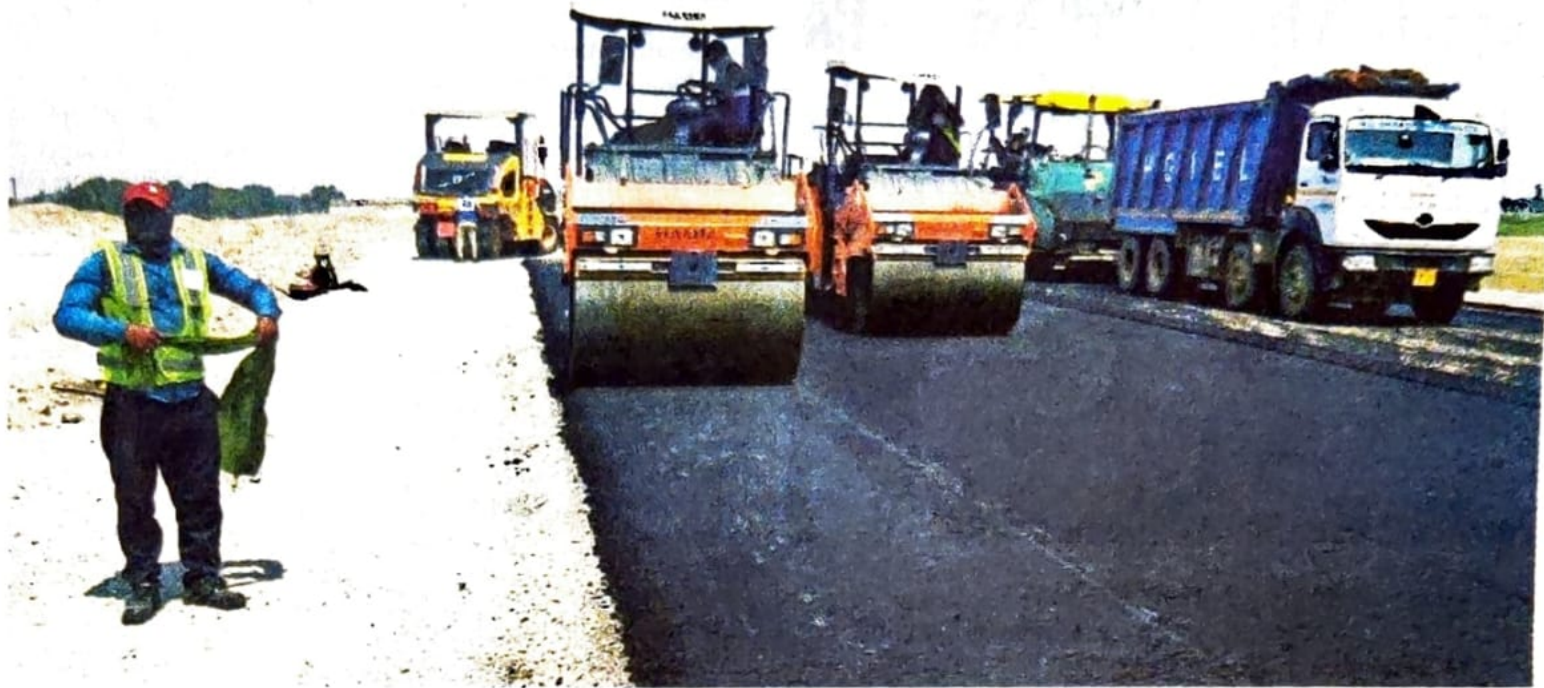
The developers have completed 25 per cent of the earthwork (scraping and grading of the patch) in just five months. Express
