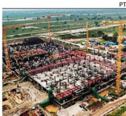
Construction work in progress at the Noida International Airport, in Gautam Budh Nagar
