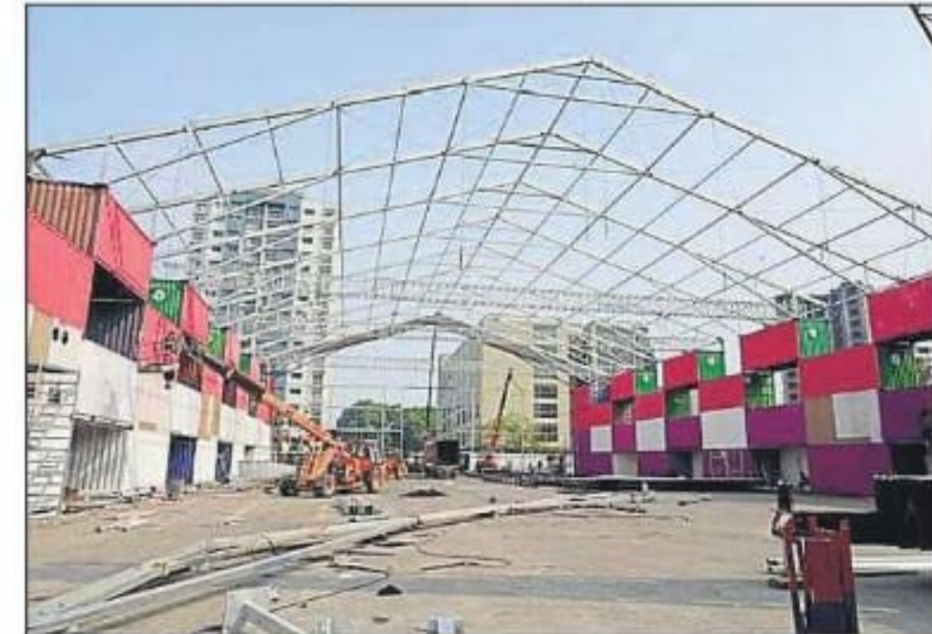
About 50 containers put up to make the grand stage for upcoming GBC 2024 at IGP on Thursday.
