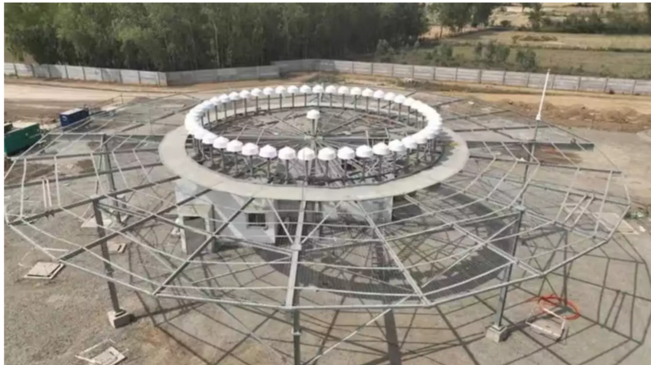
Air calibration of DVOR, DME at Noida International Airport complete
