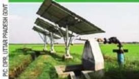
Solar pumps in UP
