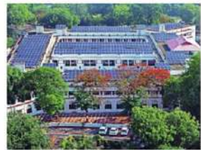
Solar panels at KGMU building in Lucknow
