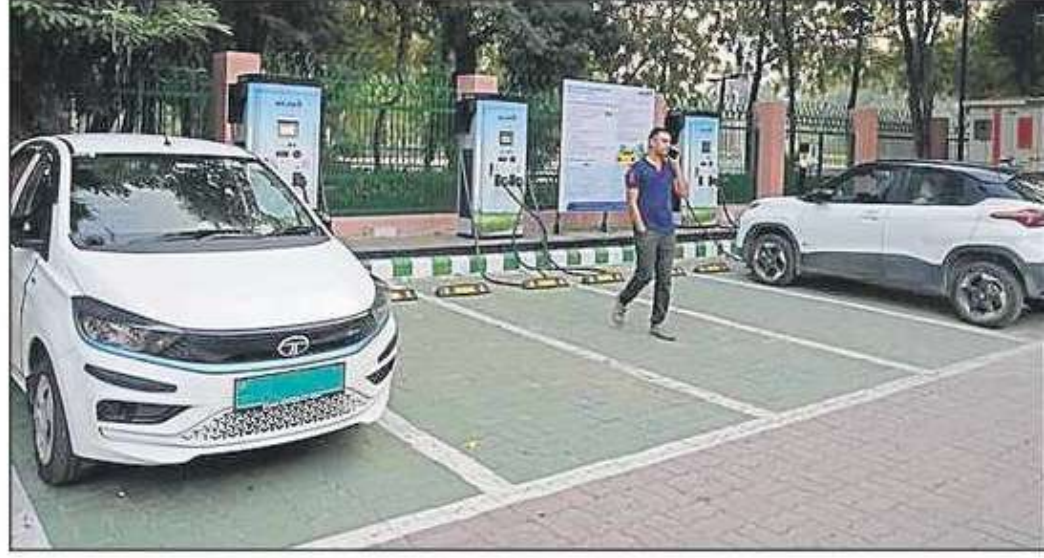
The charging station at Lohia Park in Gomti Nagar. DEEPAK GUPTA/HT
